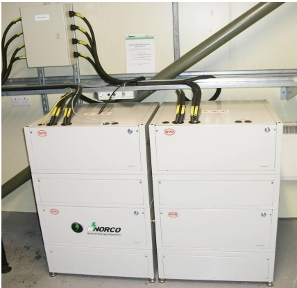
60 kWh Battery Modules
