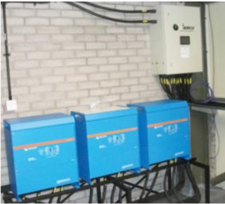
60 kW - Battery fed Inverters
