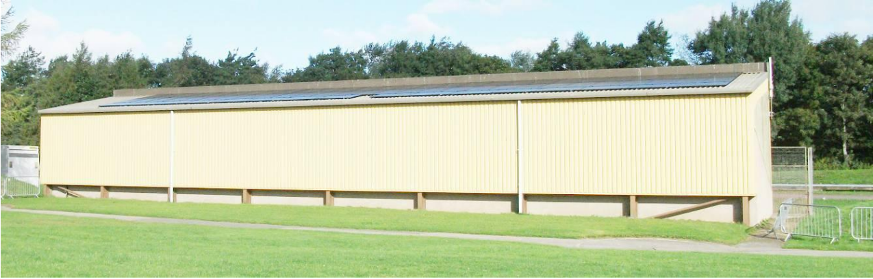
Solar PV panels mounted on Spectator Stand roof
