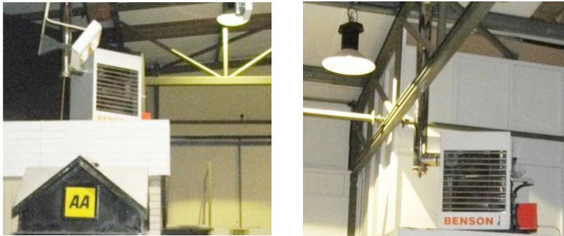
Halls 1 & 2 - Oil fired stand-by heaters
